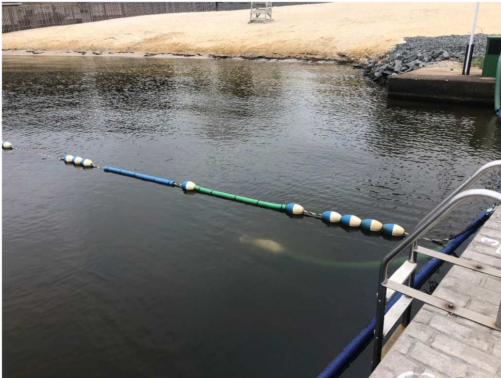
Photo 3.4 Nanobubble Oxygen System at Mt. Arlington Municipal Beach
