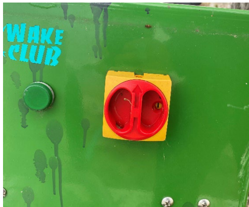
Main On / Off switch
