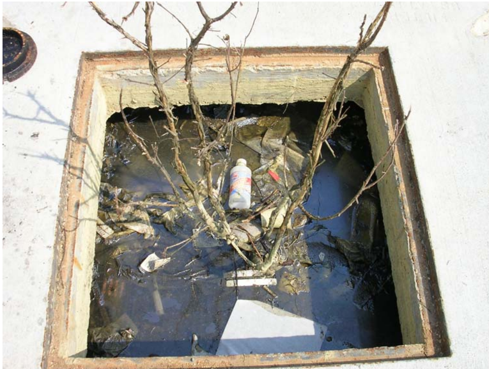
This picture shows the inside of a unit that has been neglected for several years. Filterra units are like all other stormwater BMP's and require regular maintenance to ensure they continue to operate efficiently.
