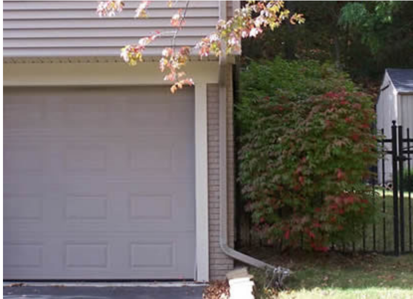
Photo 4.13: Downspout Disconnection, Source: USEPA
